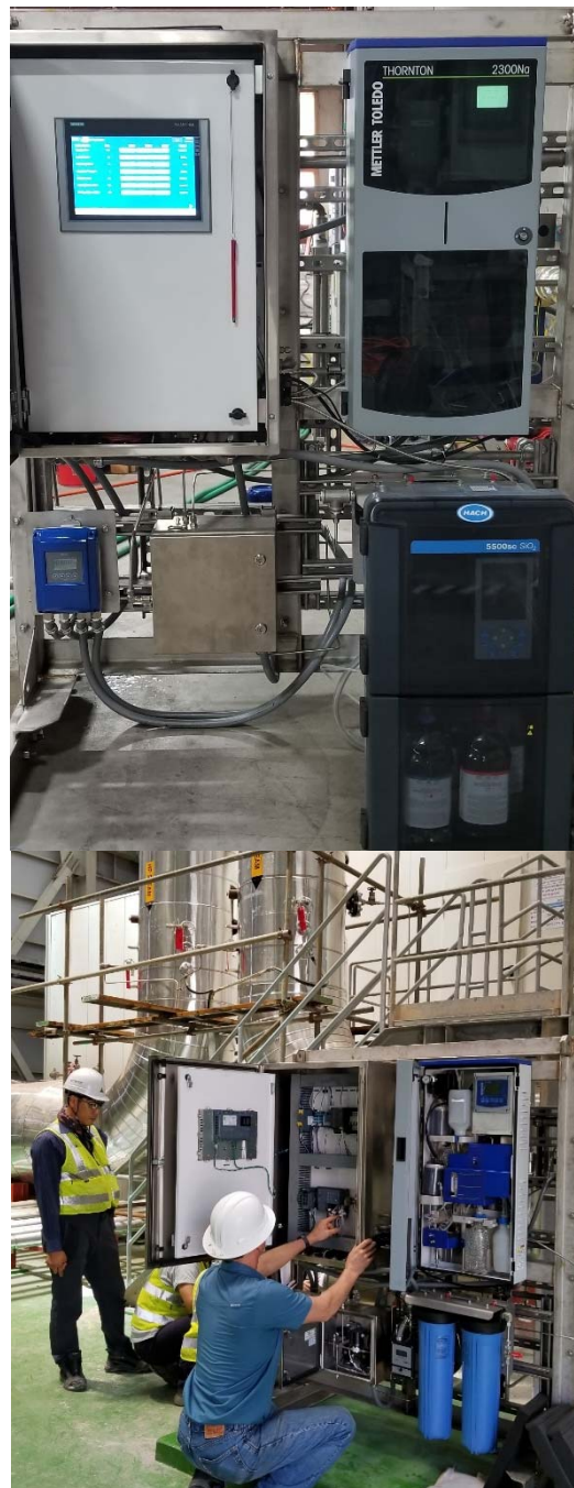
Commissioning New Steam Purity Analyzers at Silangkitang and Namora Langit Power Plants (330 MW)
